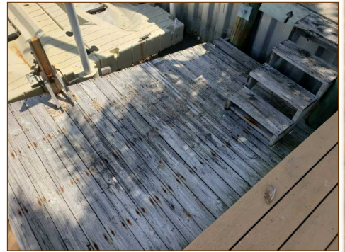
Some wood decking boards are splintered
