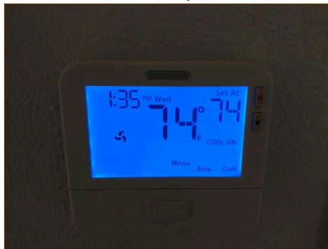
Left at 74 as found, system still running
