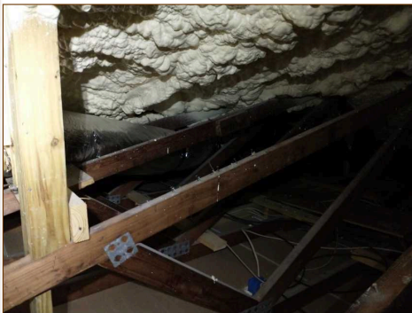
No supply ductwork in attic space
