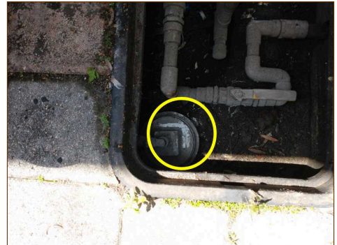
Main sewer cleanout
