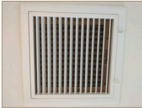
Dirty filters replaced by inspectors
