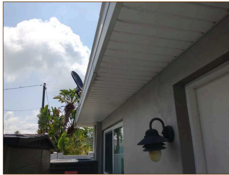
Minor moisture staining, flattened drip edge
