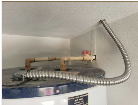
The electric service appears acceptable
