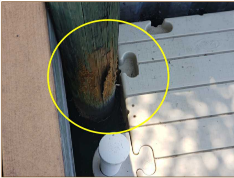
Piling in need of some repairs before use.
