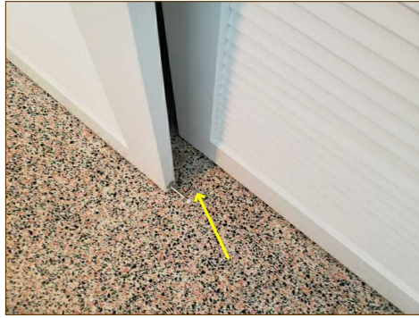
Missing bottom track guides in guest master bedroom
