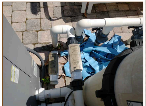
Chlorine generator cell
