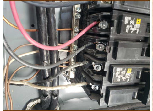
Copper branch wiring
