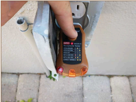
No GFCI protection
