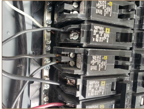
Copper branch wiring
