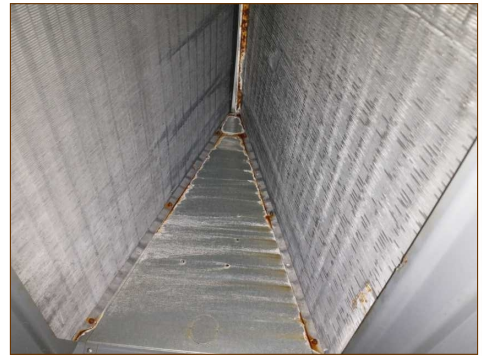
View of inside of coil, Minor accelerated wear noted
