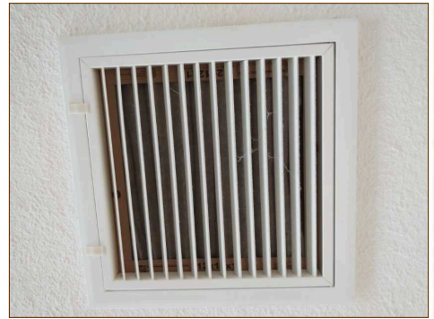
Dirty filters replaced by inspectors
