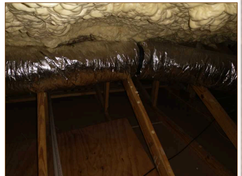
Low clearance and ductwork
