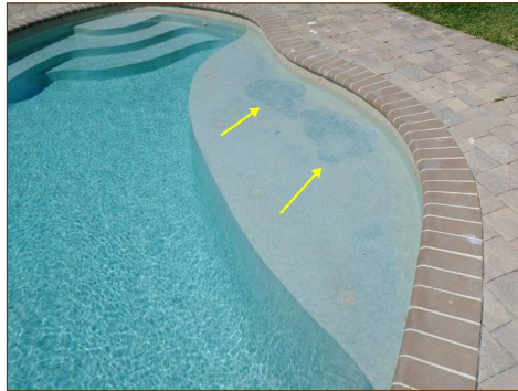
Minor staining noted
