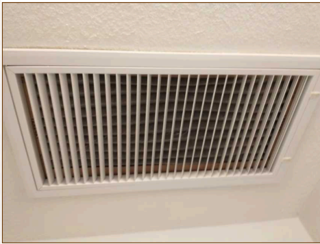
Dirty filters replaced by inspectors
