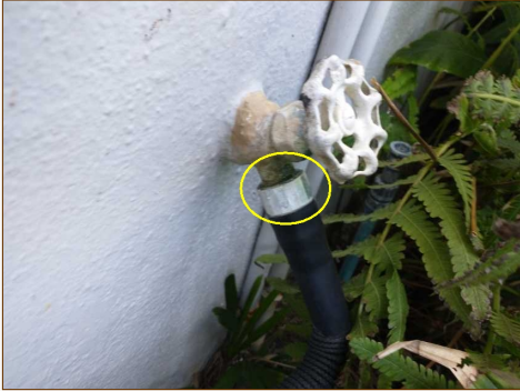
No backflow preventer(s)
