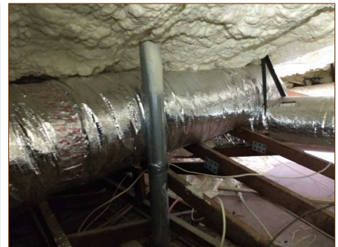
No return ductwork in attic space
