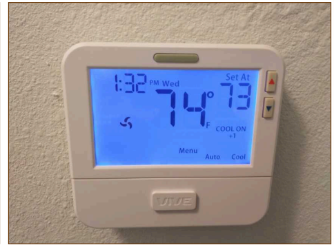
Check in, temperature dropping very slowly and system still running
