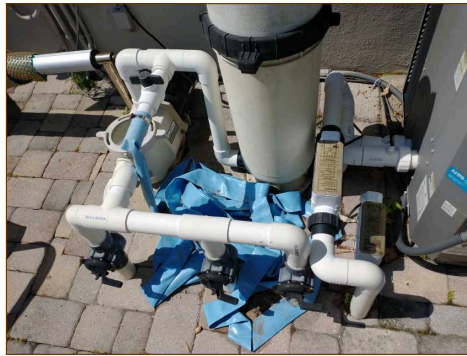
Visible plumbing in good condition
