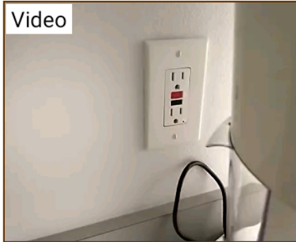
Inoperable GFCI outlet in laundry
