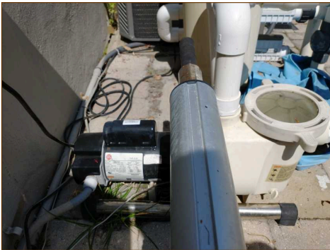
Pump and motor
