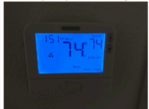
System never shut off
