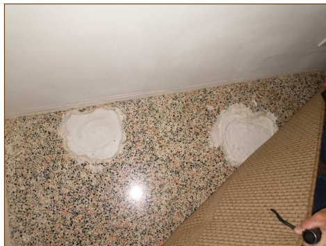
Minor damage in 2nd bedroom
