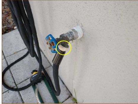
No backflow preventer(s)
