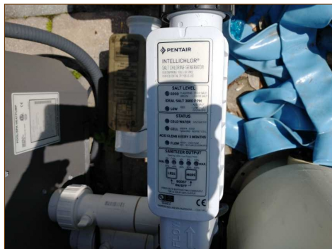
No indications illuminated on chlorine generator cell
