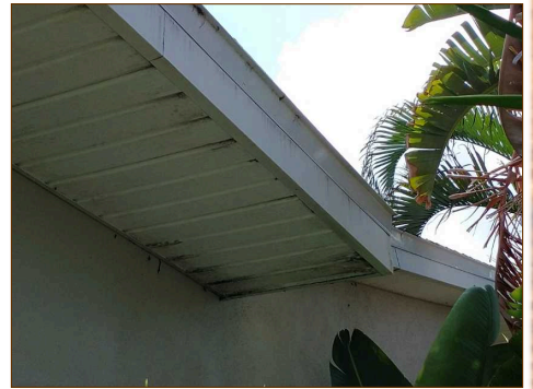
Minor moisture staining, flattened drip edge
