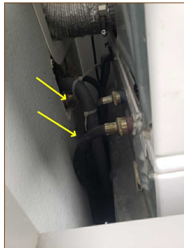
Supply hose upgrade is recommended
