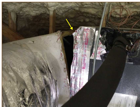
Disconnected ductwork noted, pushed together for A/C test
