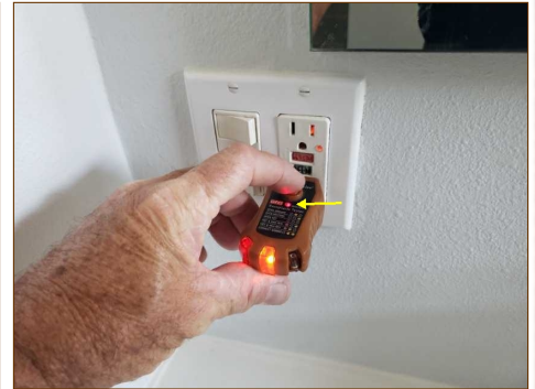
No GFCI protection in guest master suite bath
