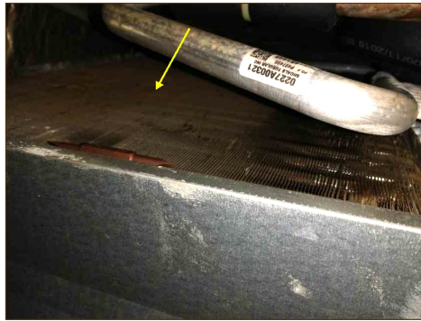
View of dirty evaporator coil
