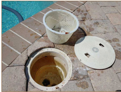
Skimmer basket in place, in good condition.
