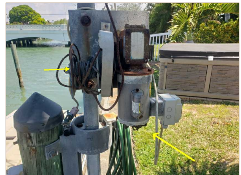
Davit lift is not operational
