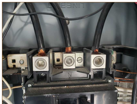
Copper entrance cables
