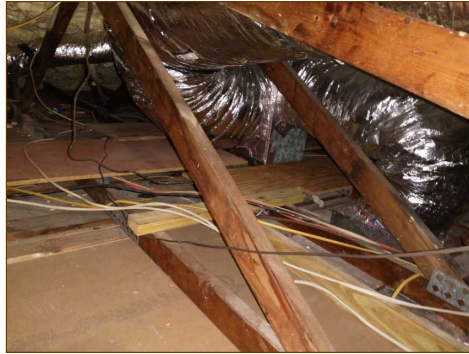
No return ductwork in attic space
