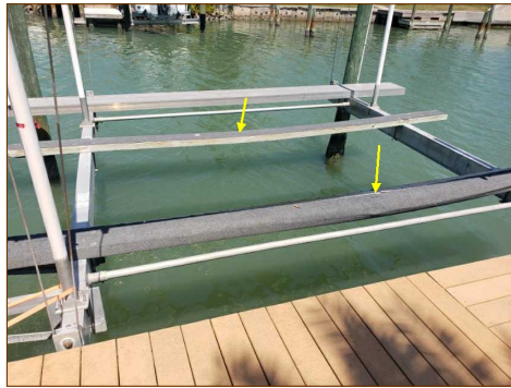
Bunks need maintenance and/or adjustment
