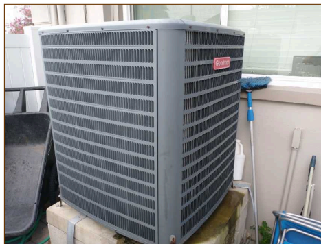
Outdoor condenser unit
