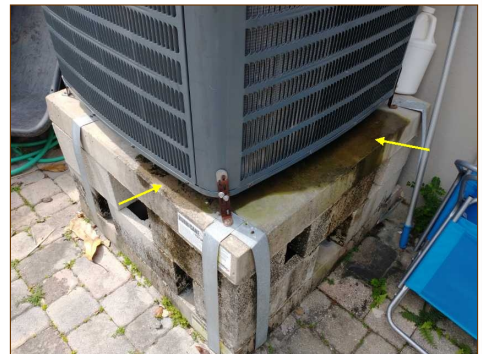
Excess condensation within unit during operation
