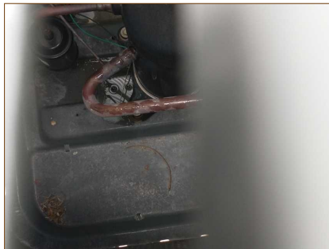
Excess condensation within unit during operation
