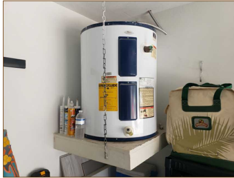
View of water heater
