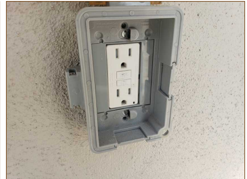
Outdoor outlets are operational and GFCI protected.
