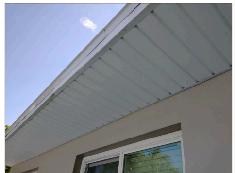
No soffit venting
