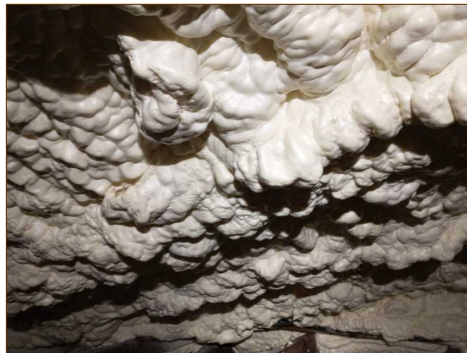
Icynene type spray foam insulation
