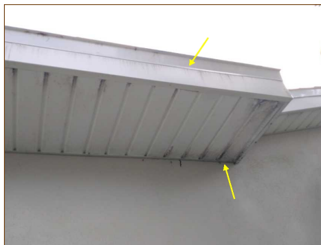
Minor staining from past leak/flattened drip edge
