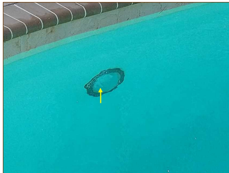
Water in pool light housing
