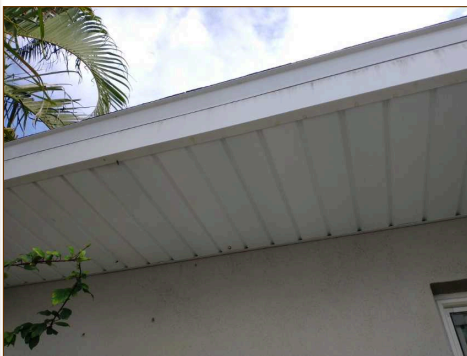
No soffit venting
