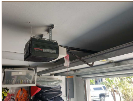
The automatic door opener is operational
