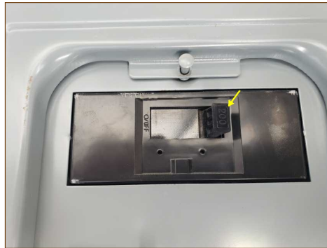
200 amp main service disconnect
